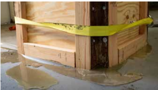
12,5000 VPM - Excessive bleed water
