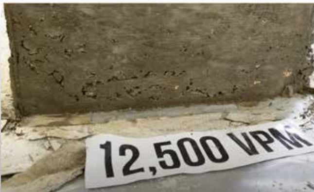
12,5000 VPM - Poor consolidation and finish
